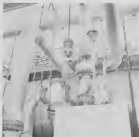
While Pipestill No. 5 is down for turnaround, Lindoro Hernandez and Jacobo Ridderstaat apply blanket-type insulation on bare fittings.
